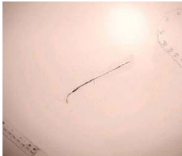
Extent of Visible Damage from Outside
